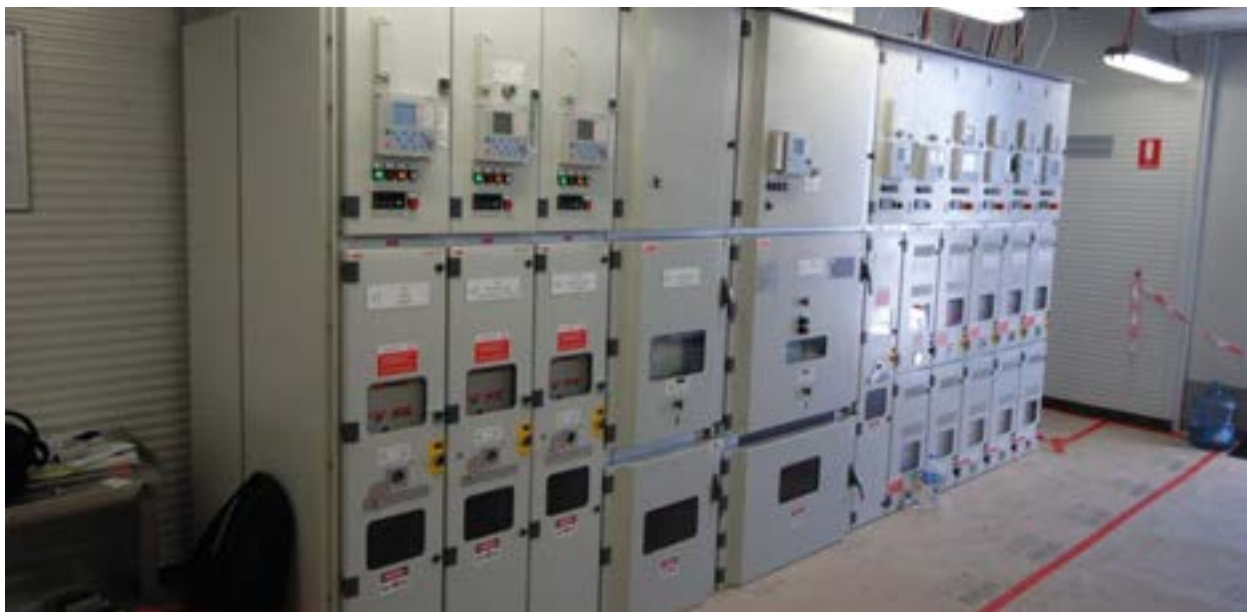
MV switchgear at LER.
