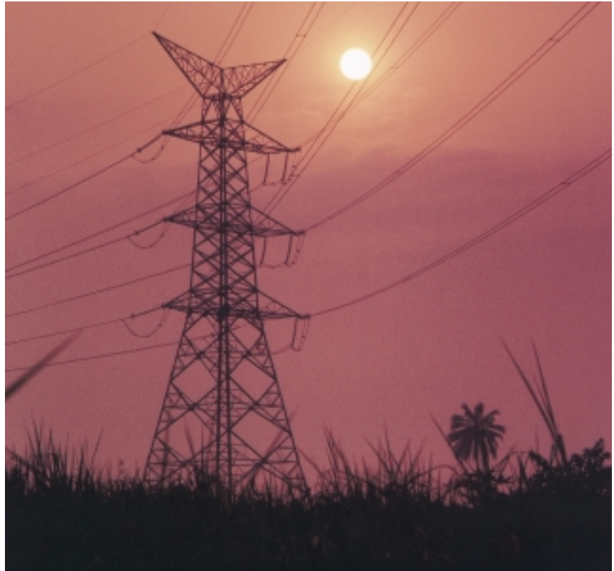
330-kV Aba-Afam double-circuit AC line, Nigeria (1982)
