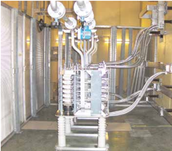
Thyristor valve (one 90 Mvar TCR branch)
