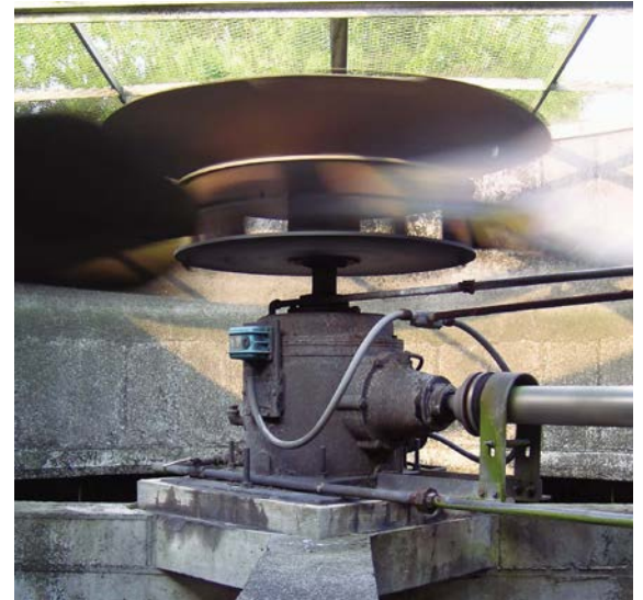
— A typical conventional fan drive arrangement of a gearbox mounted under the fan.
