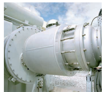
Three-phase power transformer direct connection
