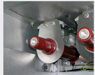
Cable termination compartment with outer cone bushings
