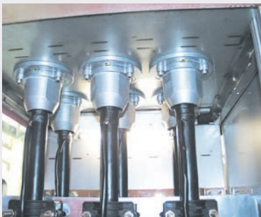
Cable termination compartment with inner cone connectors
