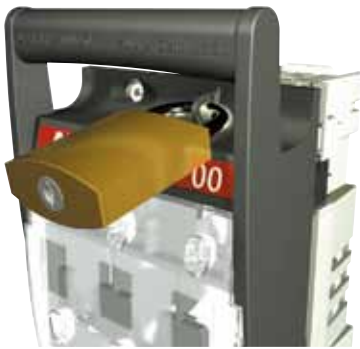
Padlocking and Sealing facilities
