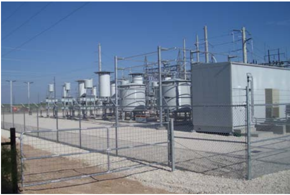
Fig. 9. Crane 69 kV, -40/+50 Mvar SVC.
