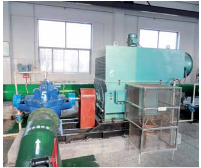
The ACS 2000 controls pump No. 5's motor, resulting in some 30 percent annual energy savings.
