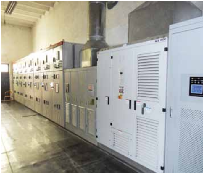
The ACS 2000's small footprint allowed the drive to be fitted within the control room's limited space.
