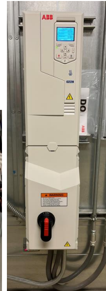
Figure 5: AHU mounted drive
