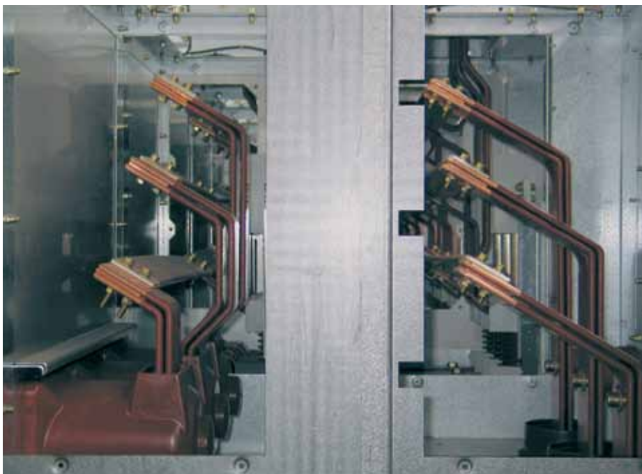
Figure 67: The two busbar compartments
