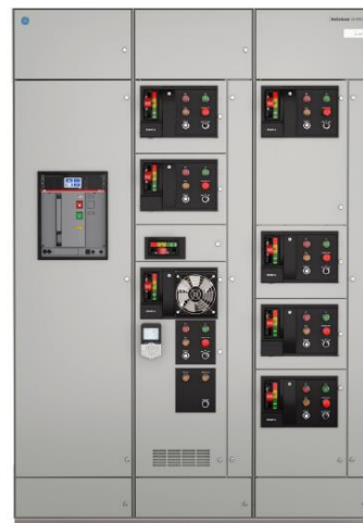
ReliaGear LV MCC
