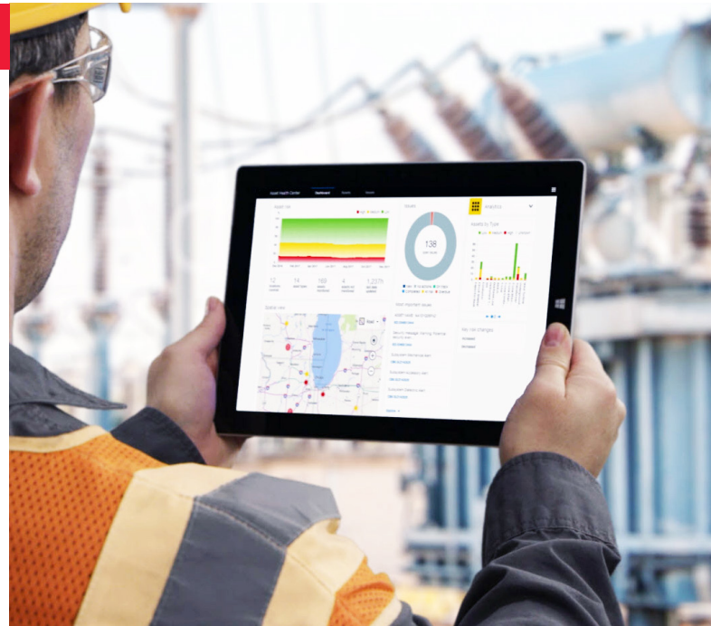
01 Online condition monitoring with CoreTec™ 4, the TXpert Hub data aggregator, is a better way to manage your transformers.
