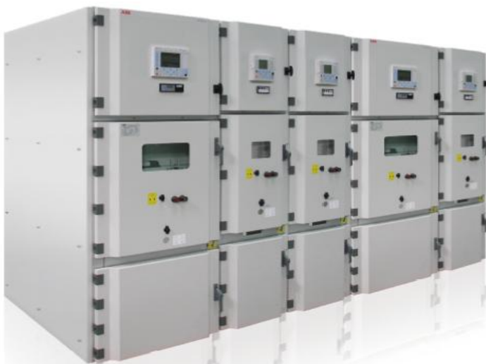
Figure 1. Typical medium voltage switchgear
