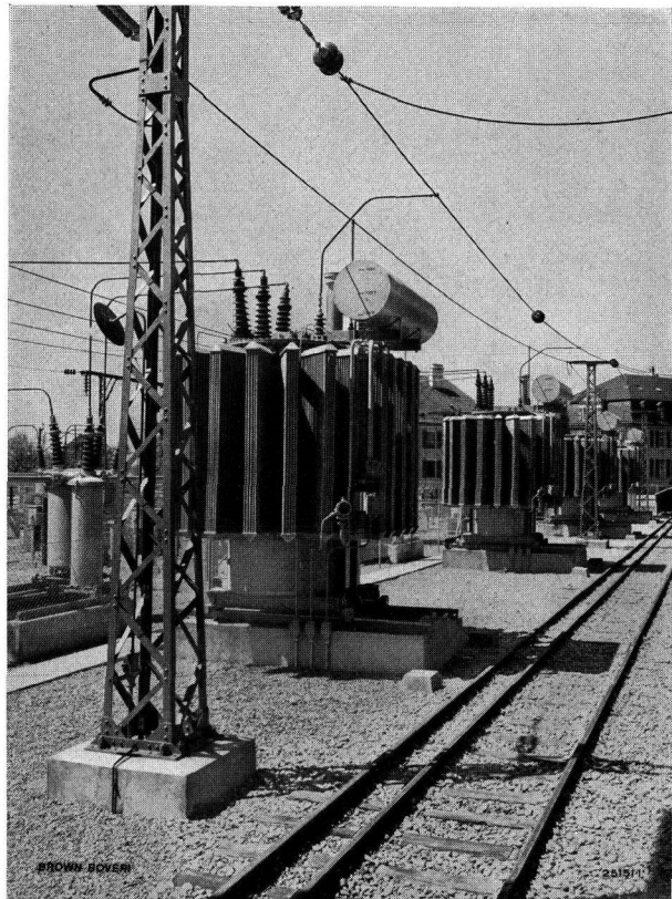
Fig. 5. — Central gangway with transformers.
