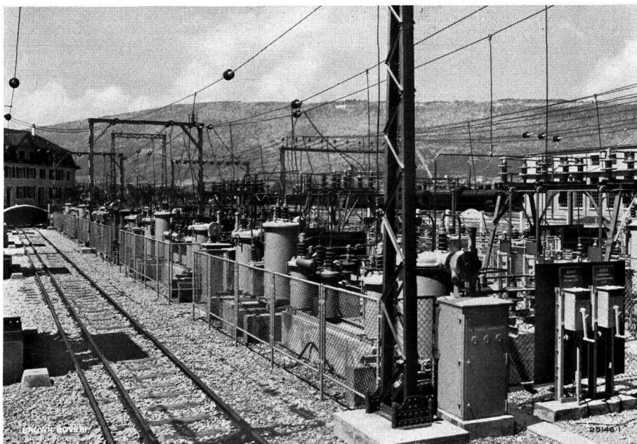
Fig. 6. — General view of the 15-kV switchgear.
