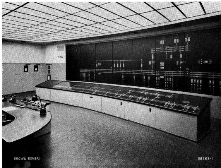
Fig. 52. — Electricity Water Works, Basle. Voltastrasse Sub-station. Control post with light diagram.
