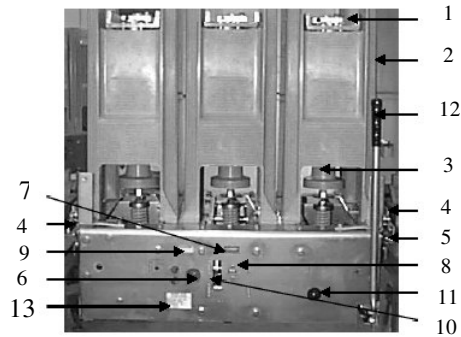
Figure 3 Front view of PowerVac breaker without front cover
