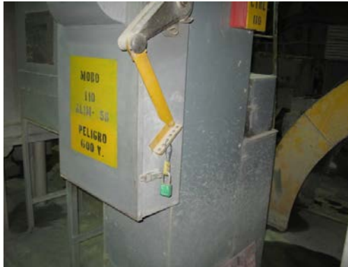
Fig 3 Lock out applied but no tag
