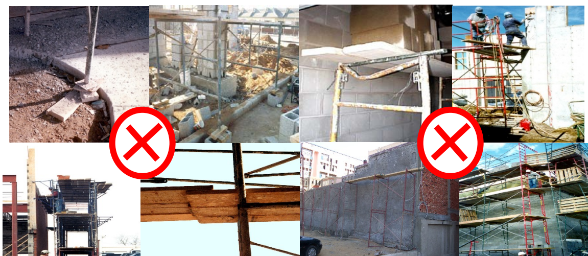
Fig 1 Examples of unsafe scaffolding-common faults
