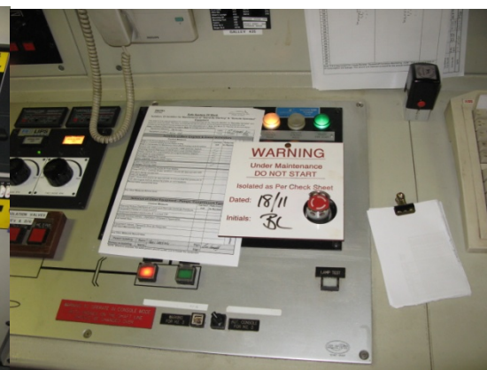
Fig 6 Control station also tagged
