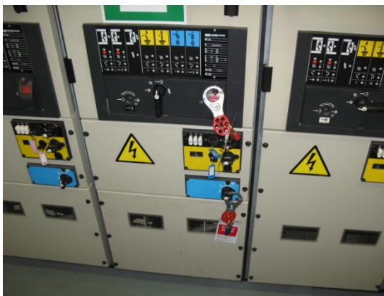
Fig 5 Panel locked out and tagged
