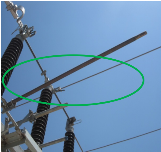
Fig 16 Earth Switch Contact at Isolator End
