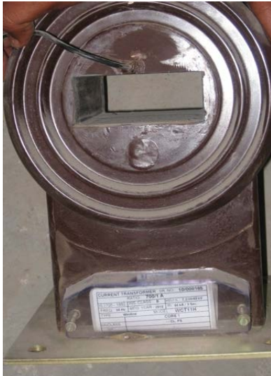
Fig 20 Secondary of Indoor Current Transformer
