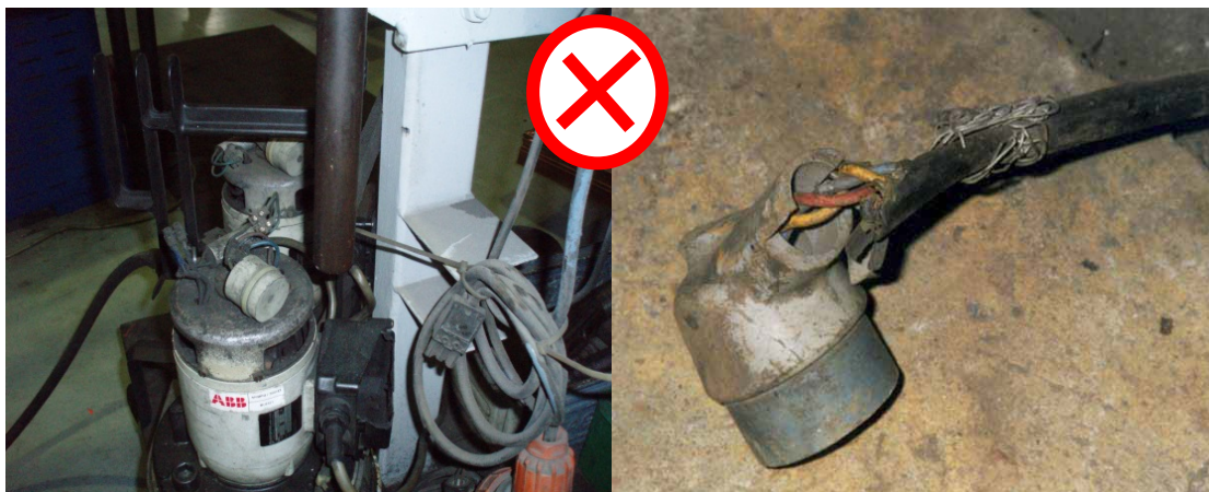
Fig 2 Examples of poorly Maintained Electrical Appliance
