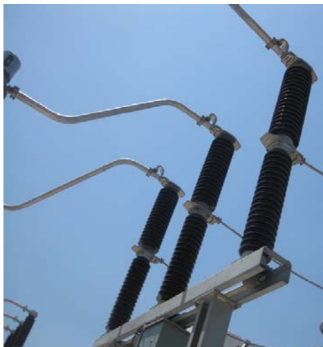
Fig 22 Outdoor Circuit Breaker
