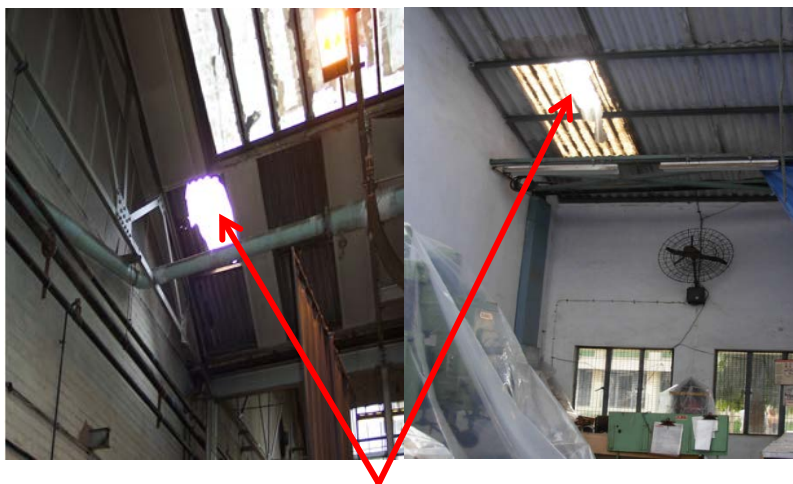
Fig 2 Broken roof lights following a person falling
