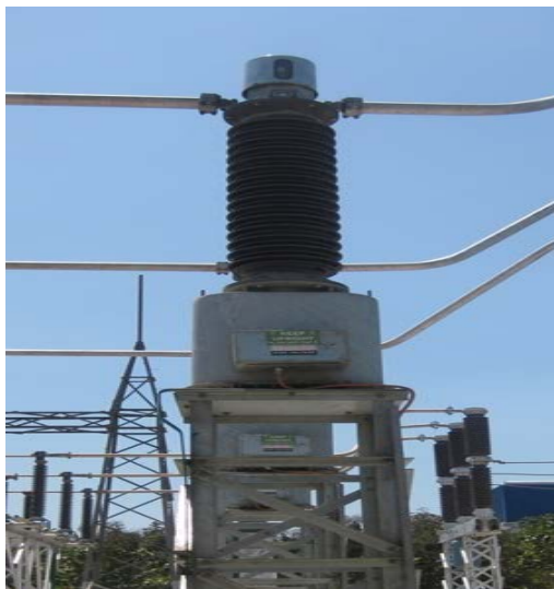
Fig 18 Outdoor Current Transformer
