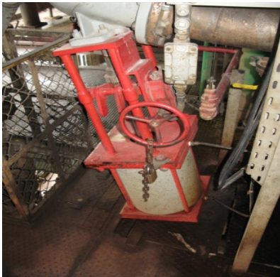
Fig 9 Valve Chained and Locked but not Tagged
