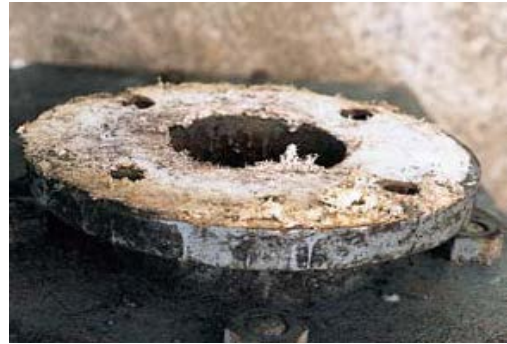
Photo 6 Remains of Asbestos from Gasket on Pipe flange
