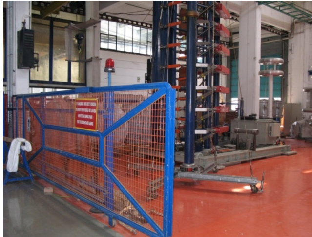
Fig 9 HV Test Area with Interlocked Gates and Fixed Barriers
