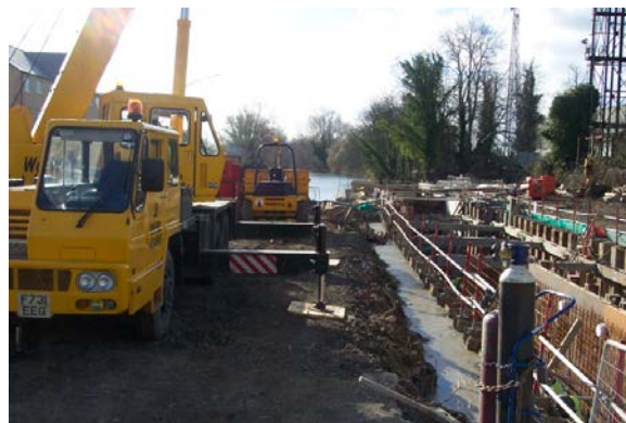
Fig 6 Correct Use of Outriggers
