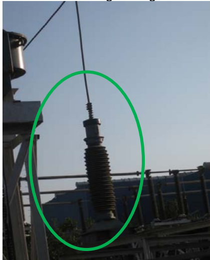
Fig 14 Outdoor Potential transformer
