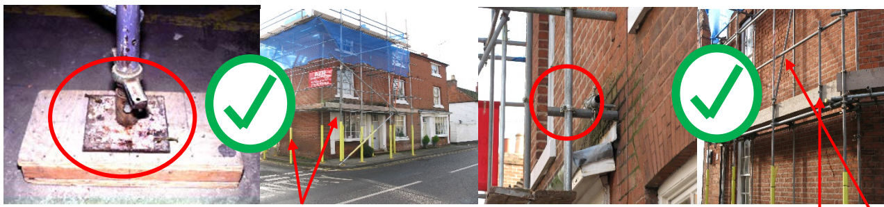
(a) Sound footing (b) Vertical uprights + bracing (c) Secured by ties (d) platform, toe boards/rails
