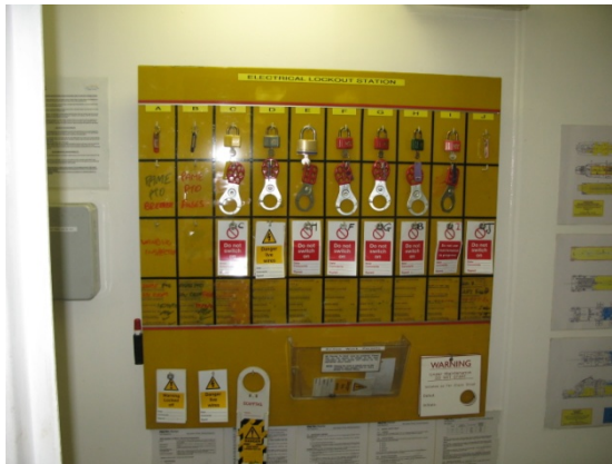
Fig 7 Control of Lock out tag out Equipment
