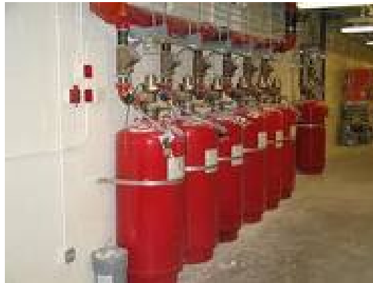
Fig 3 Automatic Fire Extinguishing System
