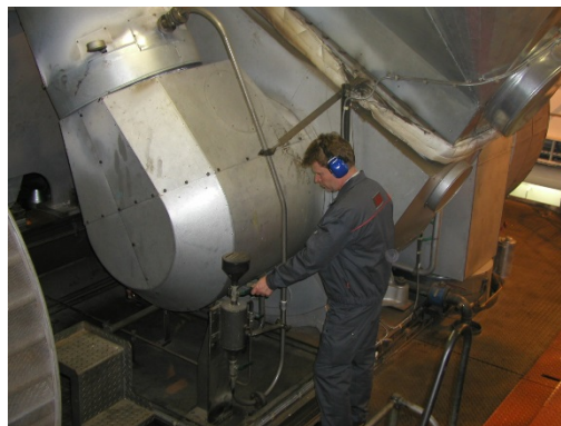
Fig 6 Hearing protection to be worn in Noise Hazard Zones
