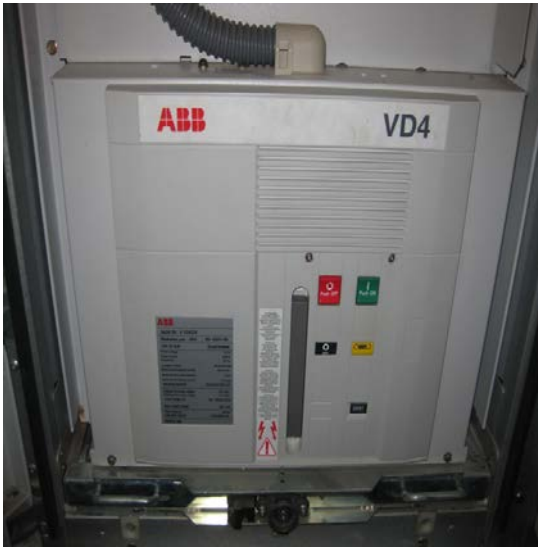
Fig 12 Indoor Circuit Breaker
