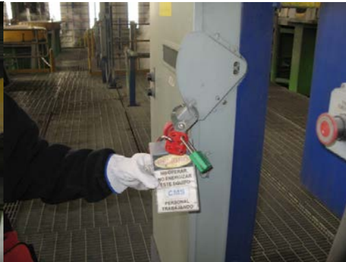
Fig 4 Locked out and tagged out
