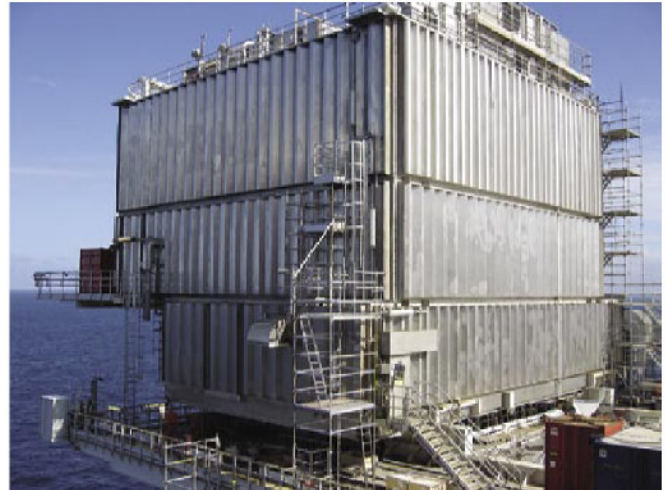
Troll A HVDC Light Unit in Position
