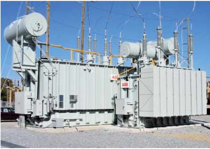
450MVA Phase shifting transformer KeySpan
