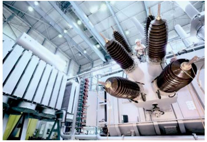
Testing of a phase shifting transformer
