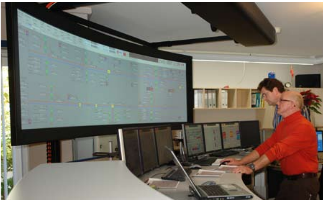
The improved modern control technology thanks to the System 800xA solution plus furnishings, including a giant screen, where the images of the different sites can be viewed and serviced, meets the approval of the operations engineers. Morten Thomsen (right) and Johnny Borgen enjoy the advantages of the new operator environment.
