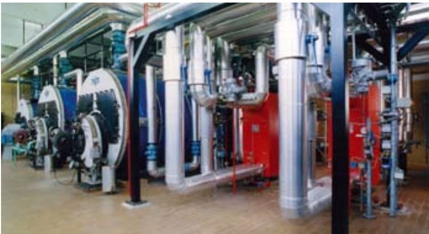
22 stations are ready to deal with heat production during peak loads. Each station is equipped and monitored by a PLC controller from ABB, which is linked in turn to the huge System 800xA based SCADA system in Fredericia.
