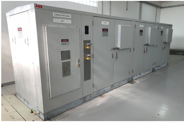
ABBACUS metal enclosed capacitor bank installed at ASRY, Bahrain
