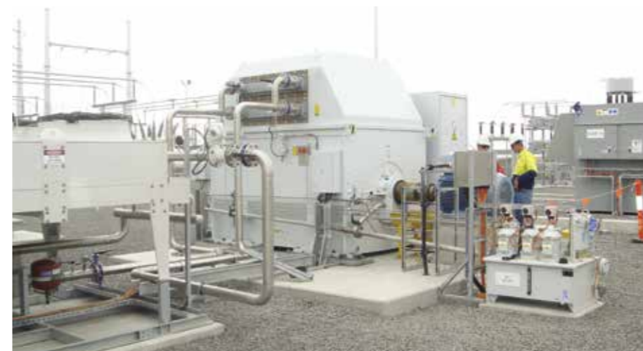
One of ABB's synchronous condensers installed in-situ.
