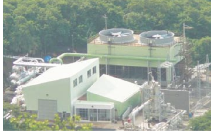
10MW Geothermal Power Plant in El Salvador
