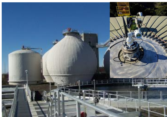
02 Digesters in wastewater treatment
