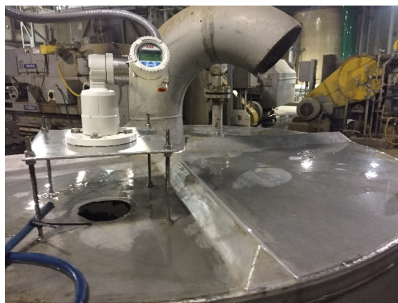
05 Control of foam level in a deaerator tank in the pulp & paper industry
