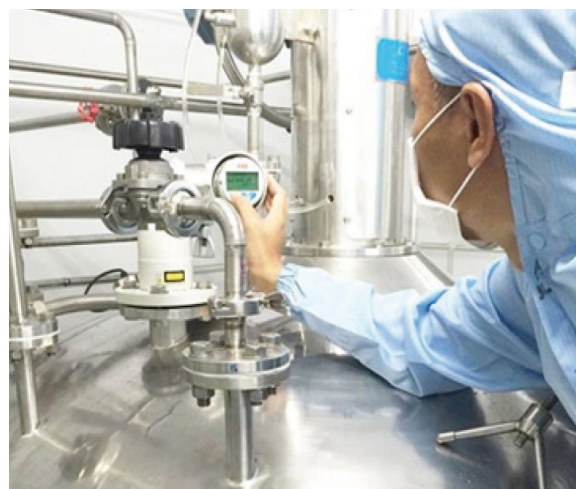
07 Foam measurement in a crystallization tank with stirrer
